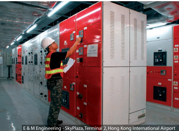
E & M Engineering - SkyPlaza, Terminal 2, Hong Kong International Airport
